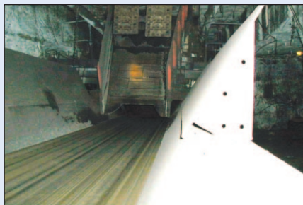
The Newstan dewatering system chute and loading station.
